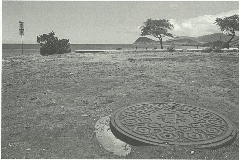
FIGURE P.1. O'ahu cable landing.
